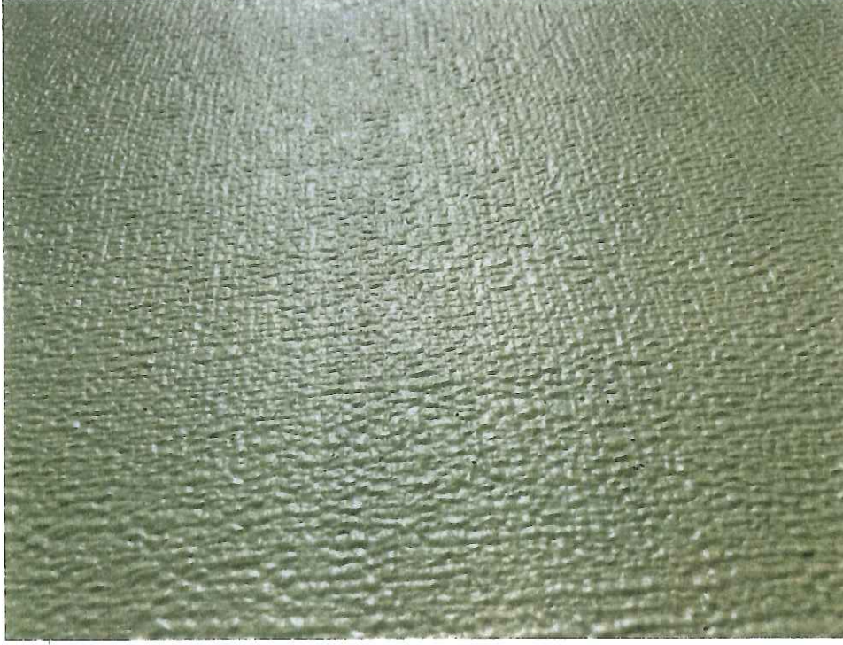
2. Closeup of Lead-Based Paint Wallpaper Texture -- Room G4
