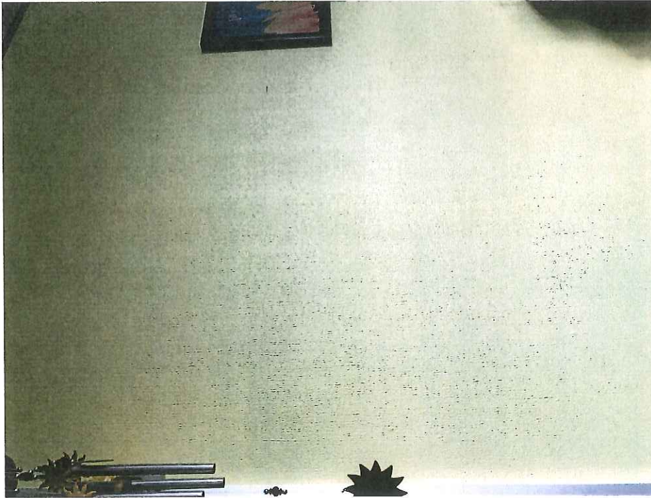
1. Wallpaper Containing Lead-Based Paint -- Room G4
